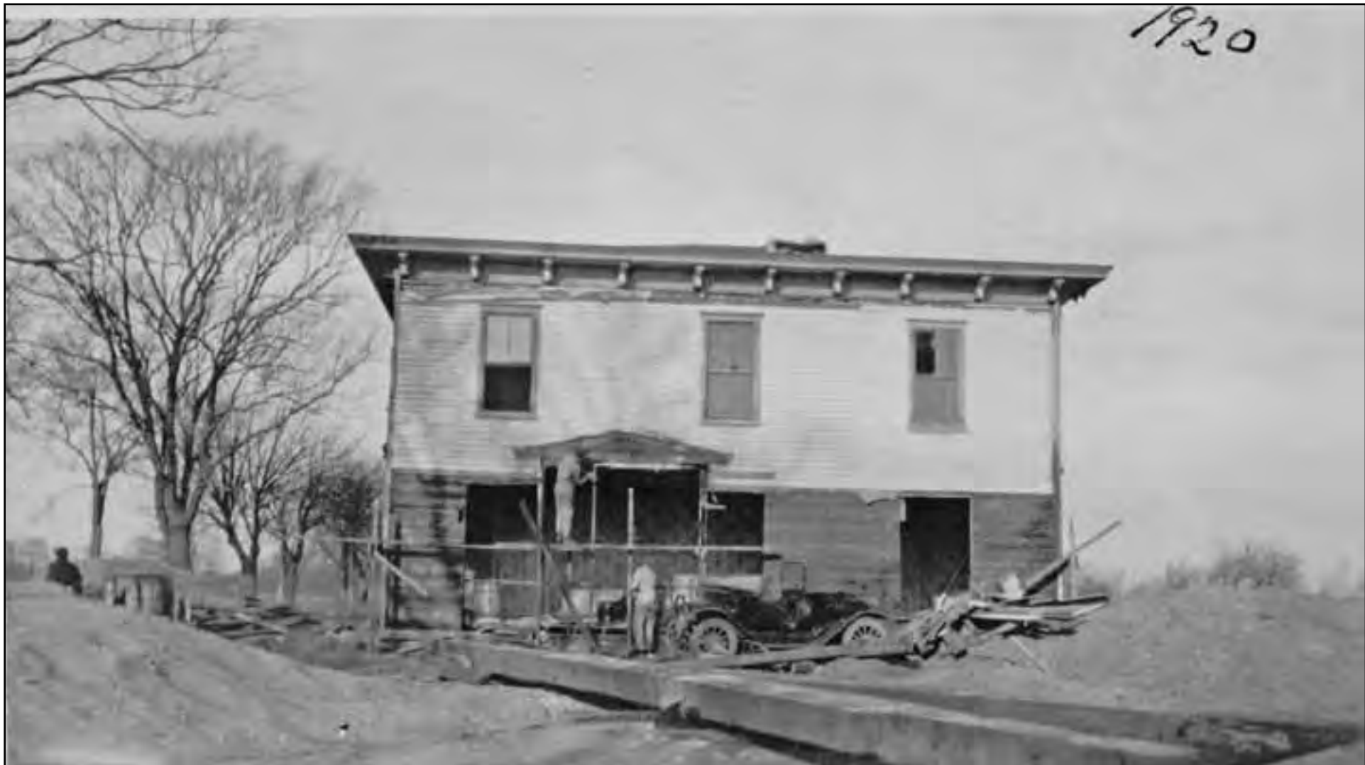
The hotel building on its new foundation. Looking northwest, the Main Road is about 1400 feet behind. The roof was lowered down once the third floor was removed. The building was turned 90 degrees to the left so that the front façade that faced the Main Road is now facing southwest. A wallpaper can be made out through the open bay window into one of the hotel drawing rooms plus two doors entering the room from the through hall. Also note the very large square timbers used as the rails to slide the house over the fields.
